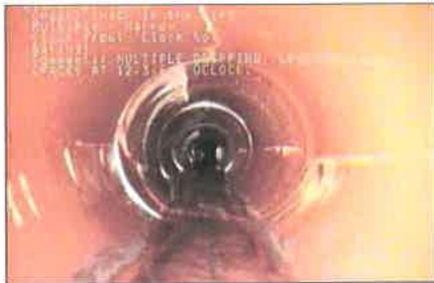
Review of televised sewer tapes showed cracked pipes and grease build-up.
